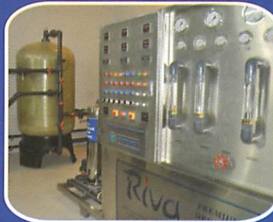
Dow "Riva" Water Filtration Plant
